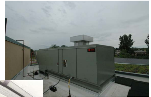
High Efficiency HVAC
